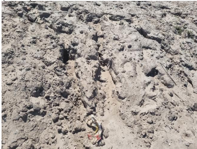
Image 5: Erosion gullies on V-drain
